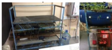
Fig.5 : Metal Rack system
